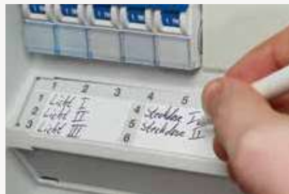
Plenty of space for circuit identification
