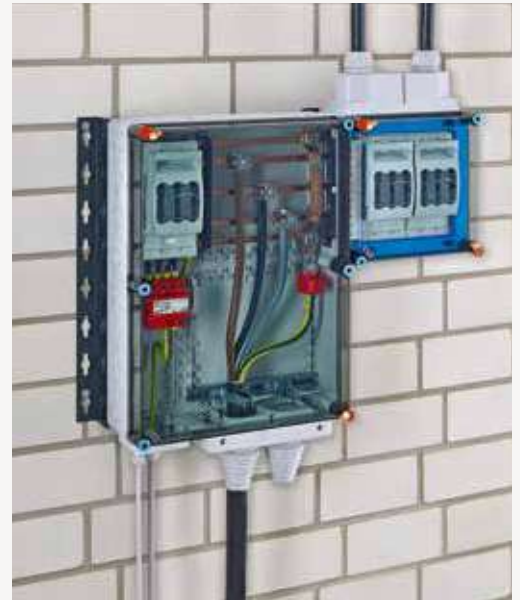
Main line distribution board for the pre-meter area
