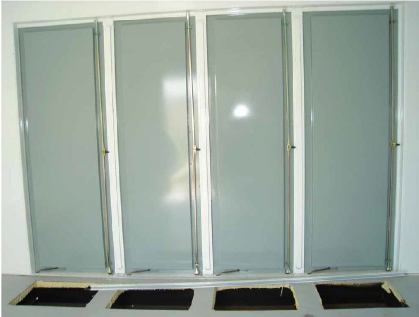
Rear Doors with Equipment conduit race cut outs
