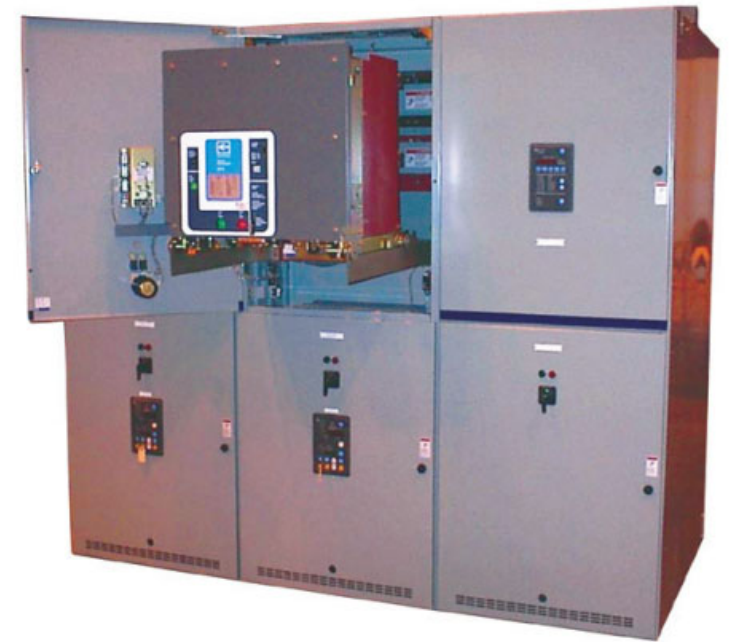
Standard Metal-Clad 5/15kV Switchgear
