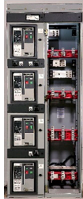
LV Metal-Enclosed Front Access 600V Switchgear
