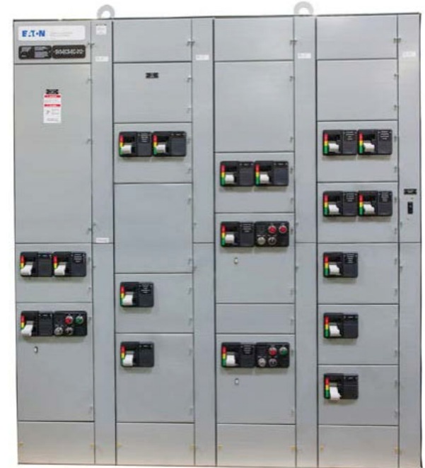
LV Motor Control Center
