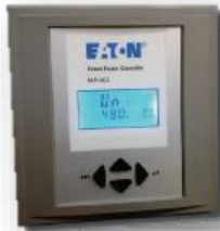
Power Factor Controller
