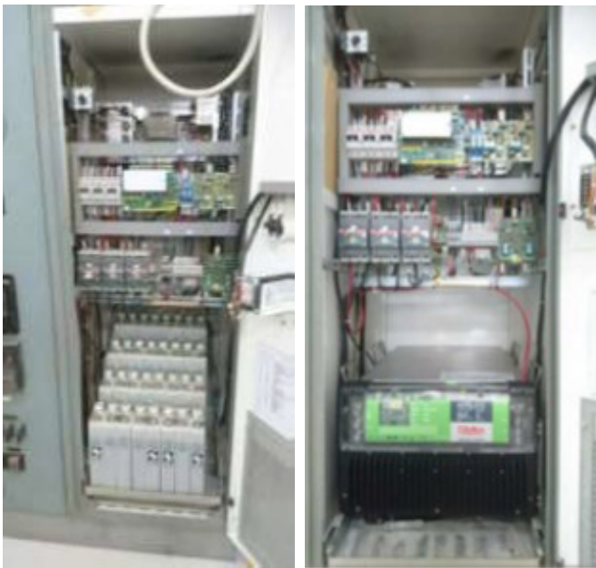
Original Battery Room with VRLA Battery
